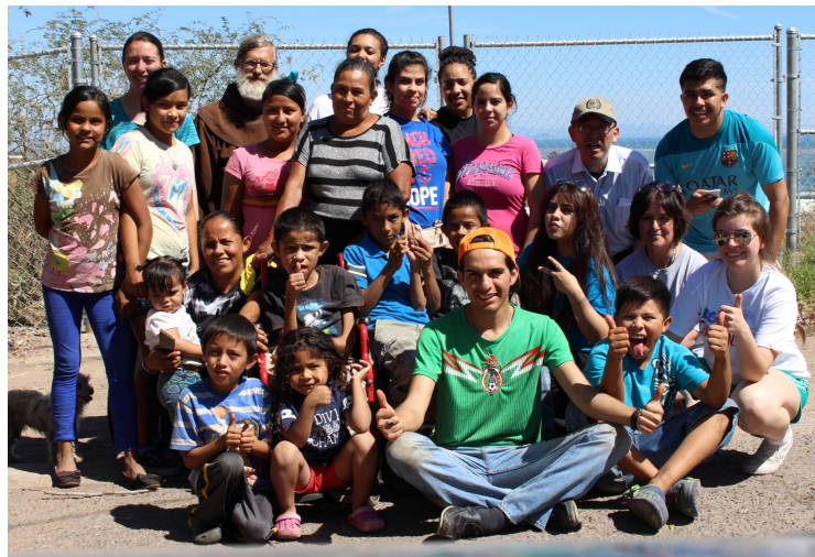
The ASU group celebrates with a family in Guaymas, after collaborating with them on a roof replacement coordinated by Casa Franciscana.
